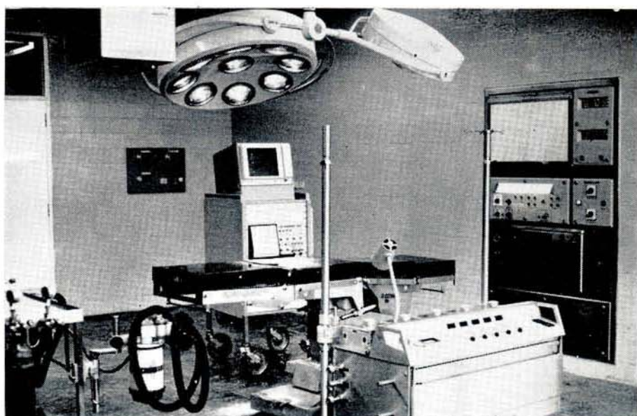
Fig. 5. The hub of the new surgical centre is the operating theatre room complex. Its total system was designed and installed by Eschmann of U. K.
